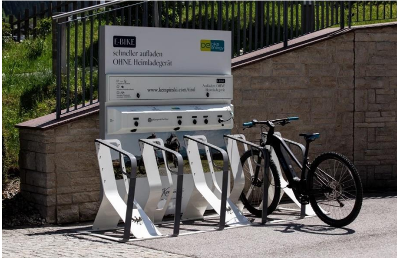
Abbildung 4 E-Bike Ladestation bike-energy
